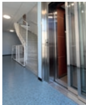
ELEVATOR INSTALLED NEXT THE STAIRWELL
